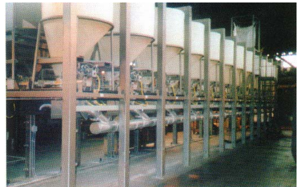
The design of the new batching system—three sloping sides paired with one shear wall—helped eliminate bridging and dust emissions.
