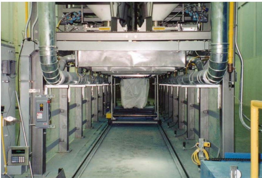
The new machine batches material directly into a super sack, enabling Morganite Crucible to keep extra inventory on hand.
